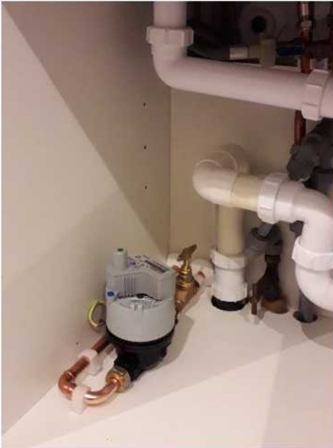
Image 5 - Internally Installed Meter
