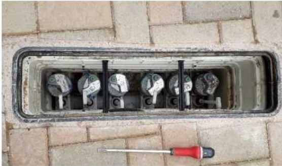
Image 3 - External (Manifold) Meter Installation
