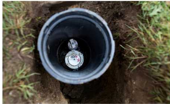
Image 4 - Externally Installed Meter
