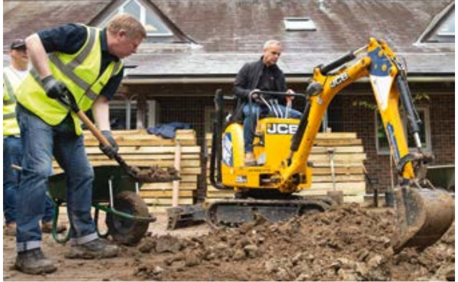
Ian Cain helping to build a water efficient sensory garden for local charity The Orpheus Centre in Godstone
